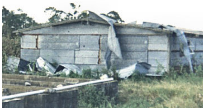
Storm damaged shed.
